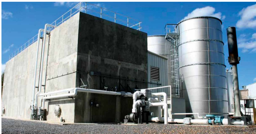
Breyers Yogurt Company installed an anaerobic treatment system at its North Lawrence Dairy to process 65,000 gallons/day of wastewater. The patented Mobilized Film Technology (reactor on left) can handle 38,000 pounds of COD/day.
